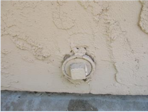
Kitchen line cleanout access
